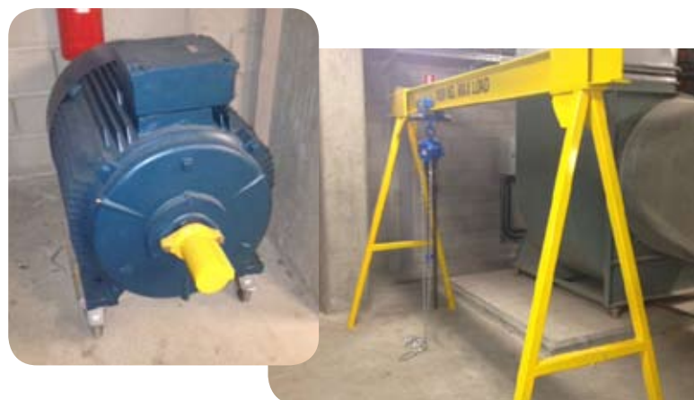
Spare equipment can be stored in convenient locations to minimise downtime, such as this condenser water pump motor and associated lifting equipment. (images courtesy of FMV)
